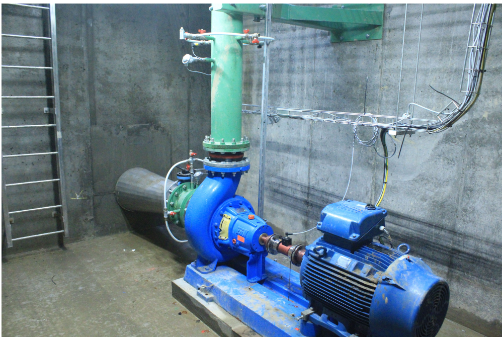
Figure 4.12: The two floors of the powerhouse or technical room of the Quartier Negundo . At the upper floor the electric panel and control system is set. In the lower floor the centrifugal PaT and the electric motor is installed.
