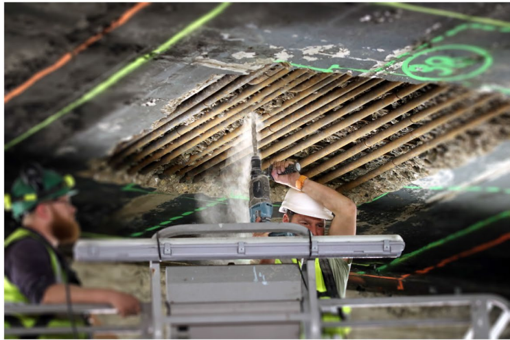
(a) A hole ( \phi 25 mm, 40 mm depth) is drilled in the ceiling (in the old concrete) between two reinforcement bars.
