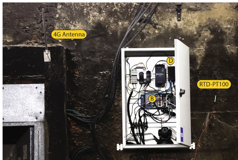
(b) Picture of the system located in the tunnel, including the 4G router.
