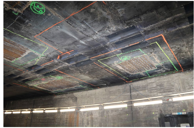
Fig. 2 General view of the zone to repair studied in the present paper. The concrete in bad state has been removed by hydro demolition
