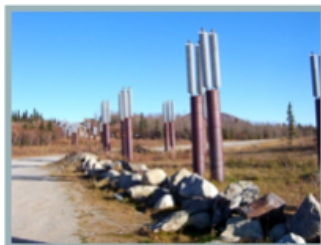
Figure 1.10: HPs are used to cool down underground soil layers to avoid permafrost melting during the warm season.
