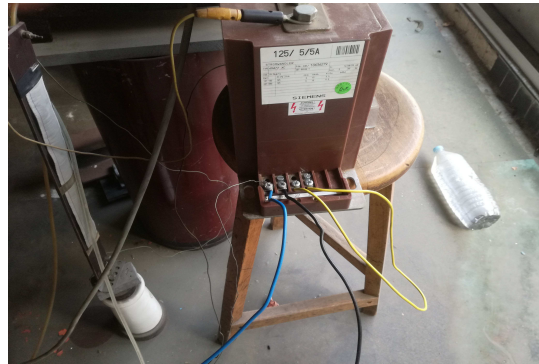
FIGURE D.6: MV CT tested during the tests.
