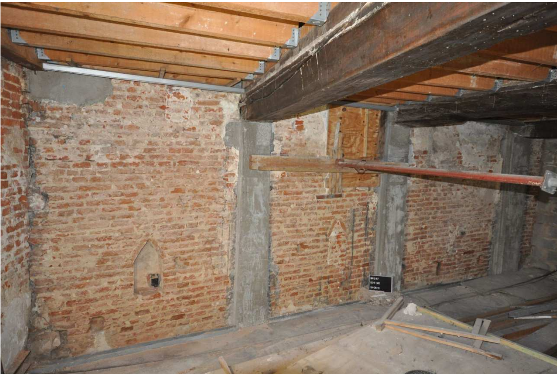
Fig. 7 – East Sidewall of the house located Rue de Flandre, no. 180, dated by AMS 14C from the period 1290-1410 (© CReAPatrimoine, ULB).
