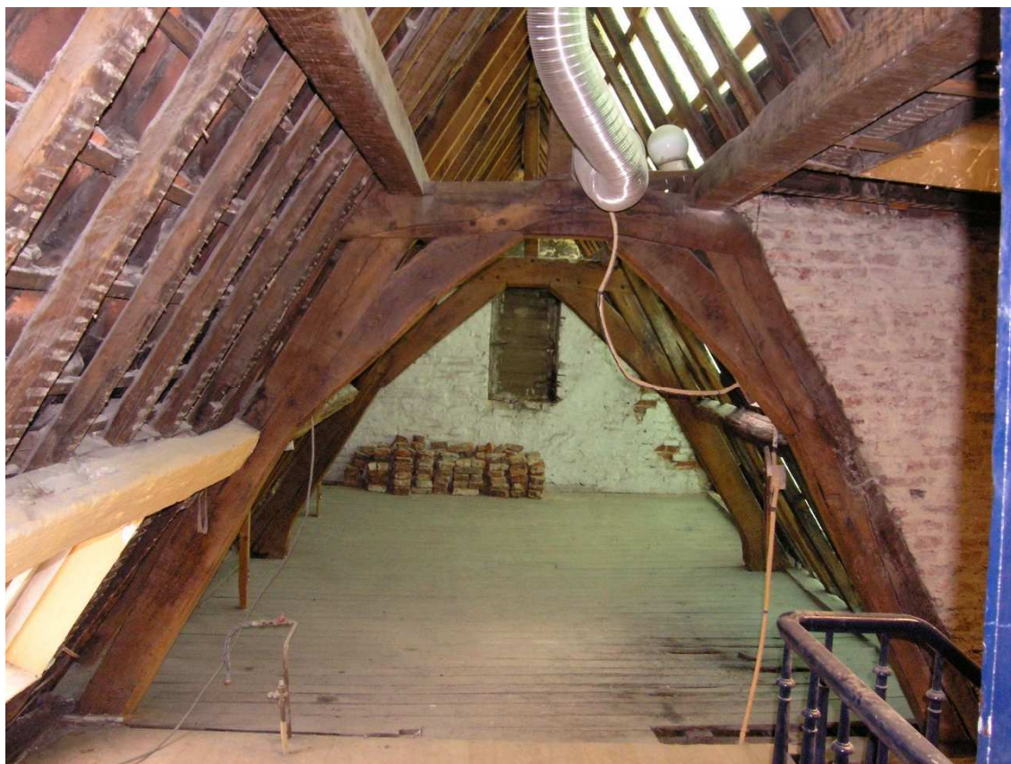
Fig. 5 – Roof frame of the back house located Rue Haute, no. 4 (© Royal Museum of Art and History, Brussels)
