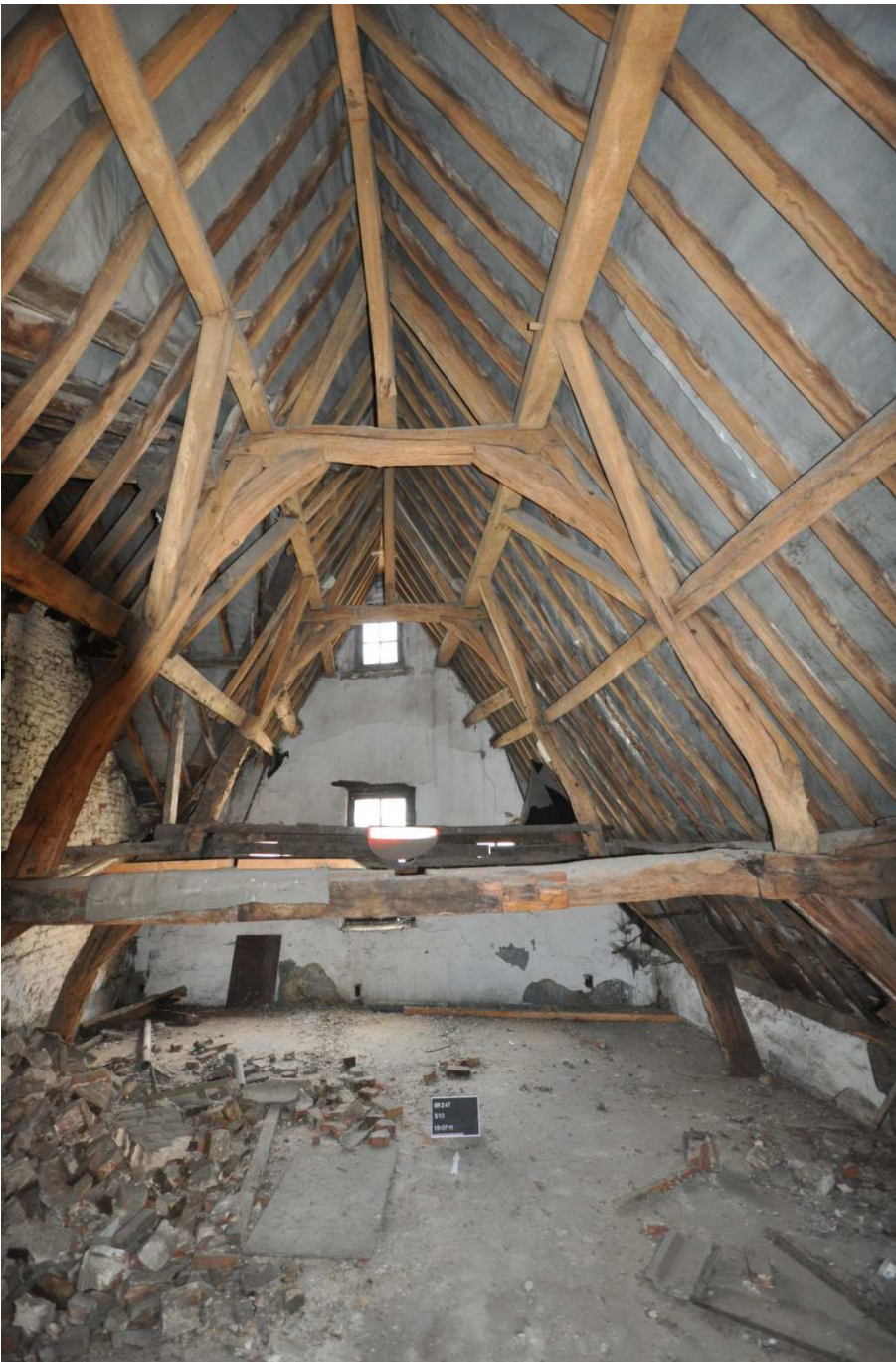
Fig. 6 – Roof frame of the house located Rue de Flandre, no. 180, dated by AMS 14C from the period 1390-1450 (© CReA-Patrimoine, ULB)
